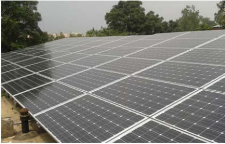
Figure 2: Parking area after installation of solar panel.
